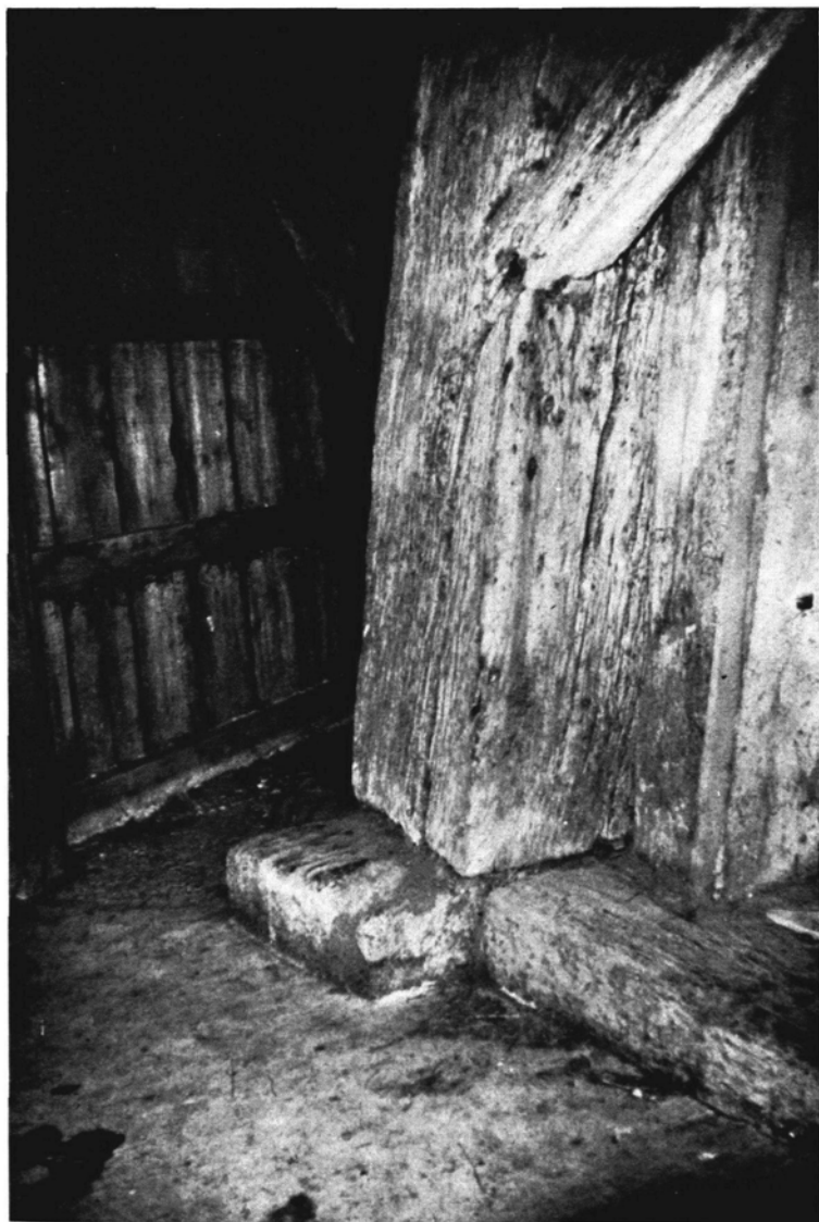
Brookland Belfry. Foot of the north-west Post, showing notched-lap Joint, at the lower end of a diagonal Brace.
